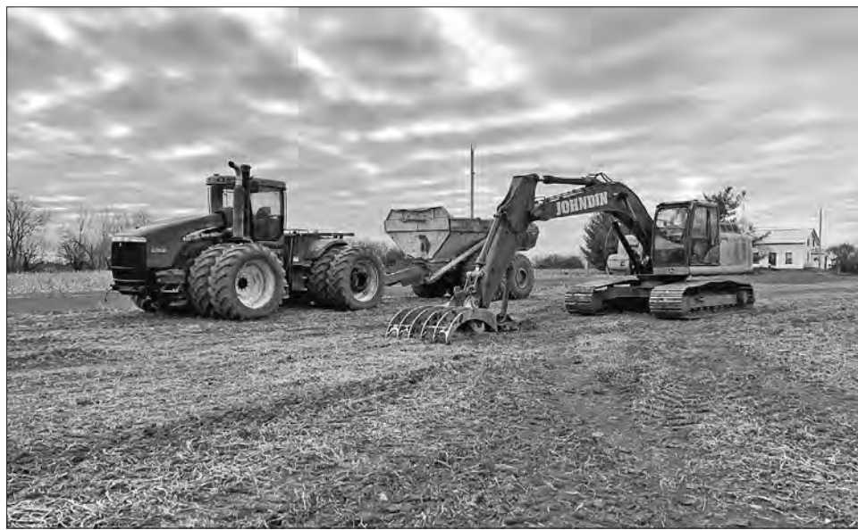
LD Excavation and Demo may be a new company but they do not lack in their experience and drive to complete the tasks you need. Courtesy Photo
